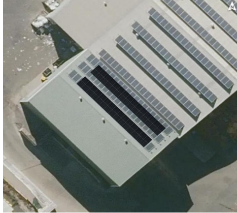
FIGURE 108: FOREST RD LANDFILL – SMRF – 15 kW FLUSH-MOUNTED ROOF SOLAR PV SYSTEM REPLACEMENT W/ 30 kWh BESS
