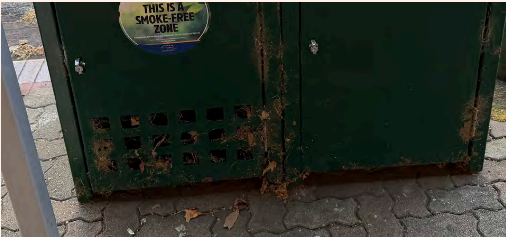
Dirty bin surround - dirt & cobwebs
